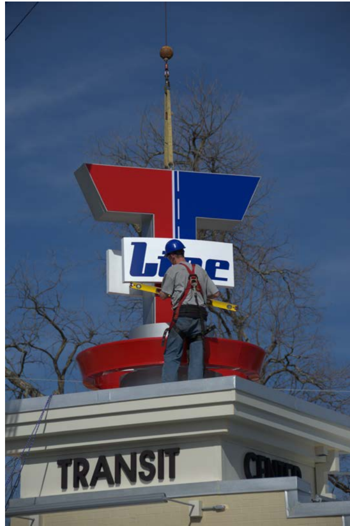
The Sign has been sat into place and is now being leveled to be bolted down
